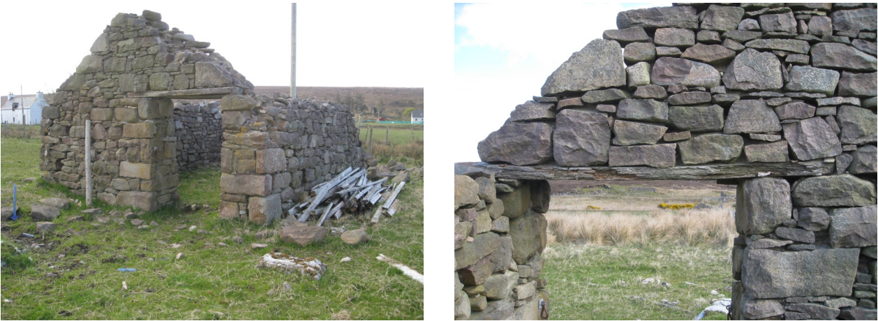
8 NG 74818 71167 30m ruined barn
