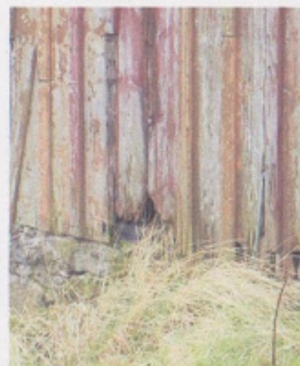
Rubble found & rotten boards
