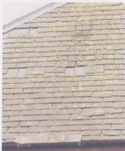
Slates slipping or missing
