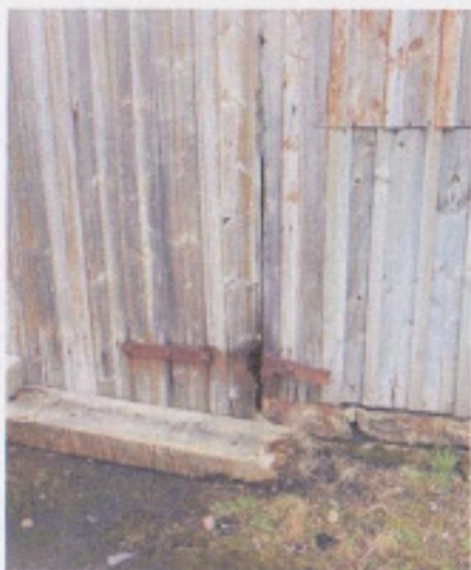
Broken Hinge & deteriorating found
