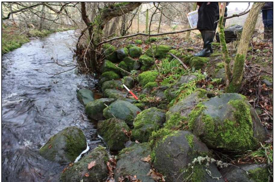
Site 5, the site of the bridge over the Peffery Burn with the remains of the abutment on the west bank
